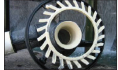
Sulfur fouling on and in the spray nozzles results in uneven water distribution over the fill.
