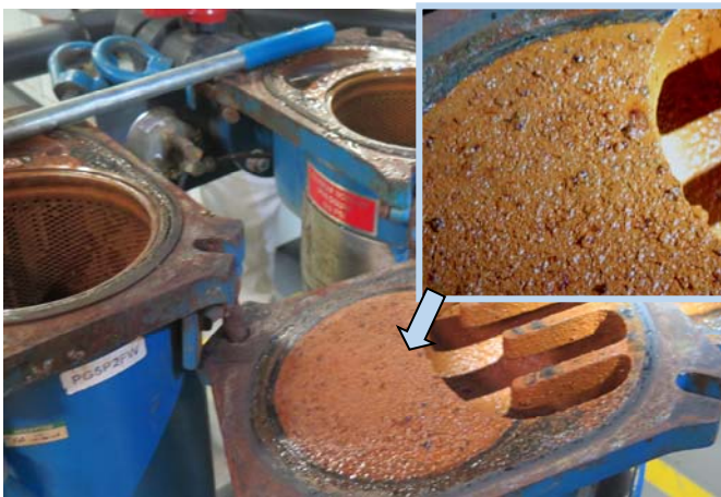
Image 1: Deposits in the housing of the filter bag system.
